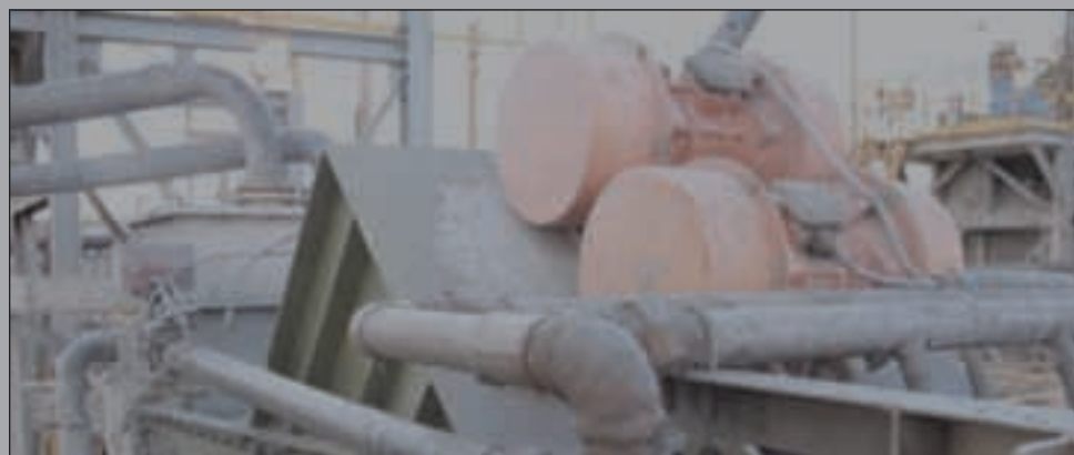
Vibrators on the refurbished KCGM screen
